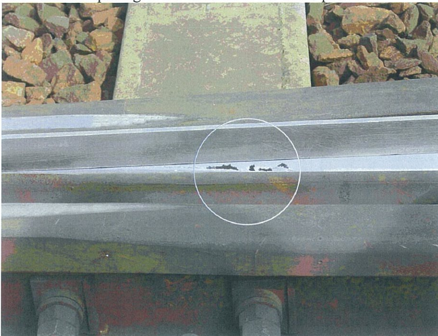
B.5 Surface spalling of the material in the initial phase.
